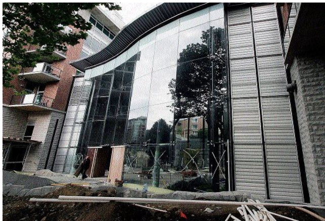
Parkside Resort and Spa's atrium will shelter a variety of plants from the former Crystal Garden.
